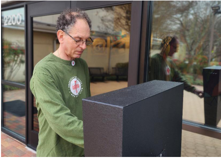
Security Committee member Jonathan Solomon checks out the newly installed building access control box.
